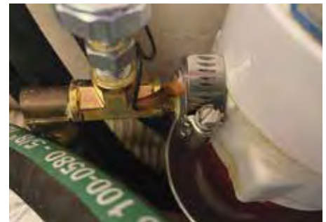
Ground wire and pressure sensor placement
