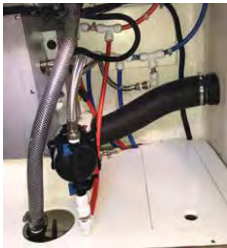
New water heater installed and the PEX supply manifold complete. The small, black tank in the center foreground is an accumulator tank.
