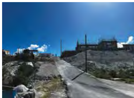
Construction underway atop the hill that leads to Duncan Town on Ragged Island.
