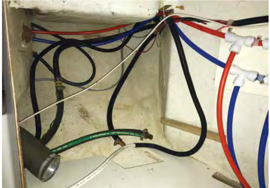
Water heater and supply pump removed and the beginning of the new PEX manifold. Note the engine heat hose running to the upper right - this would go away as part of project creep.
