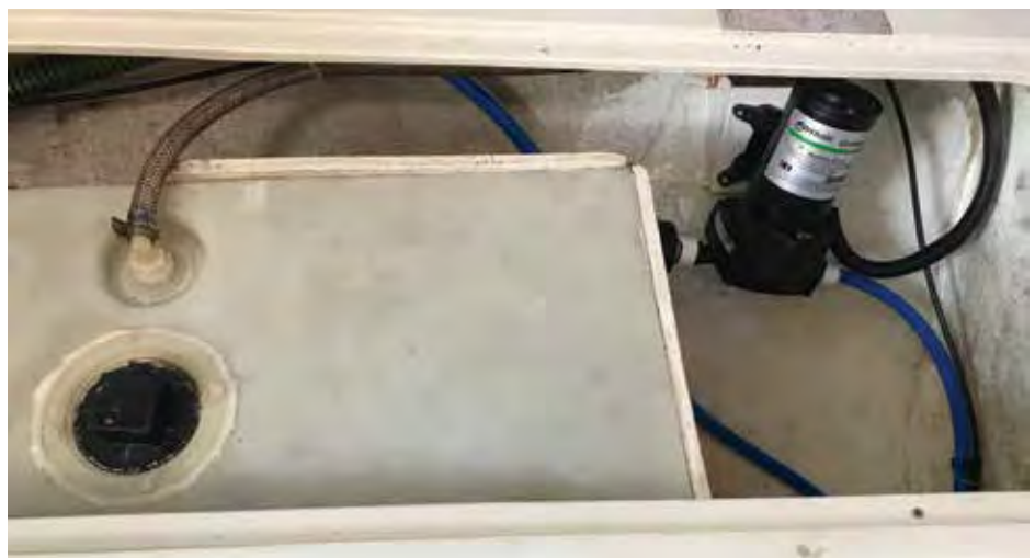
New location for the water supply pump.
