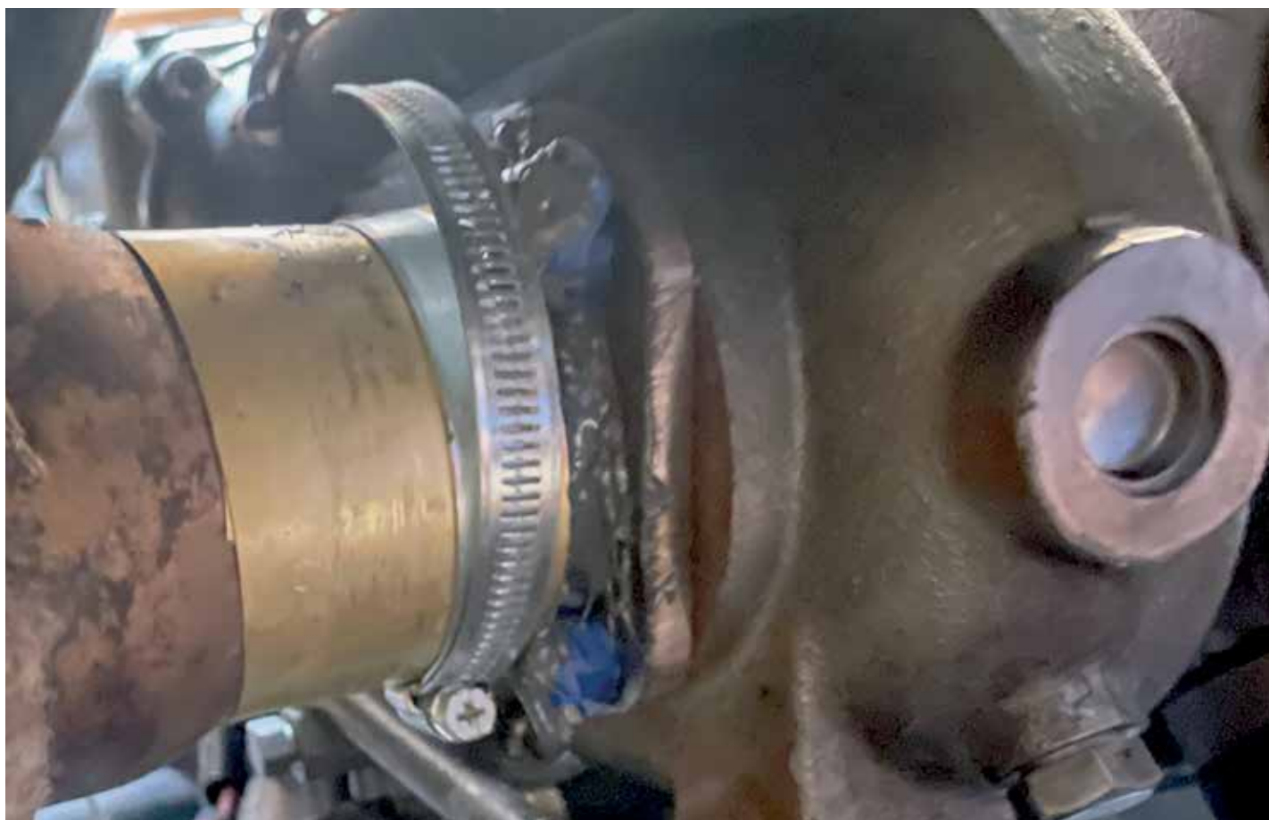
Exhaust Elbow -- Attempted Emergency Repair
