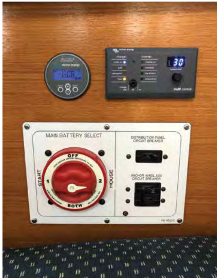
Victron BMV and Control Panel
