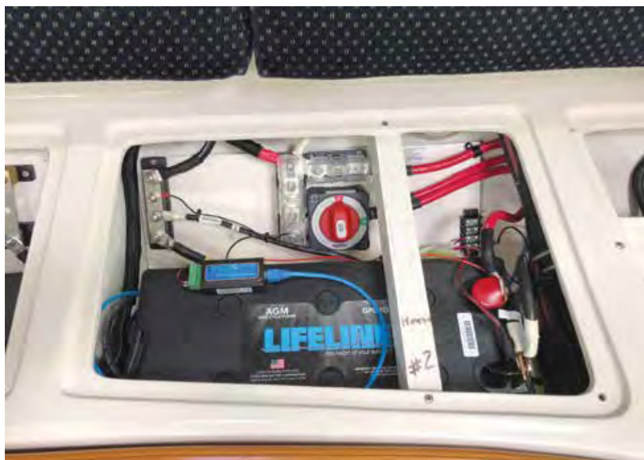
Aft Battery Compartment
