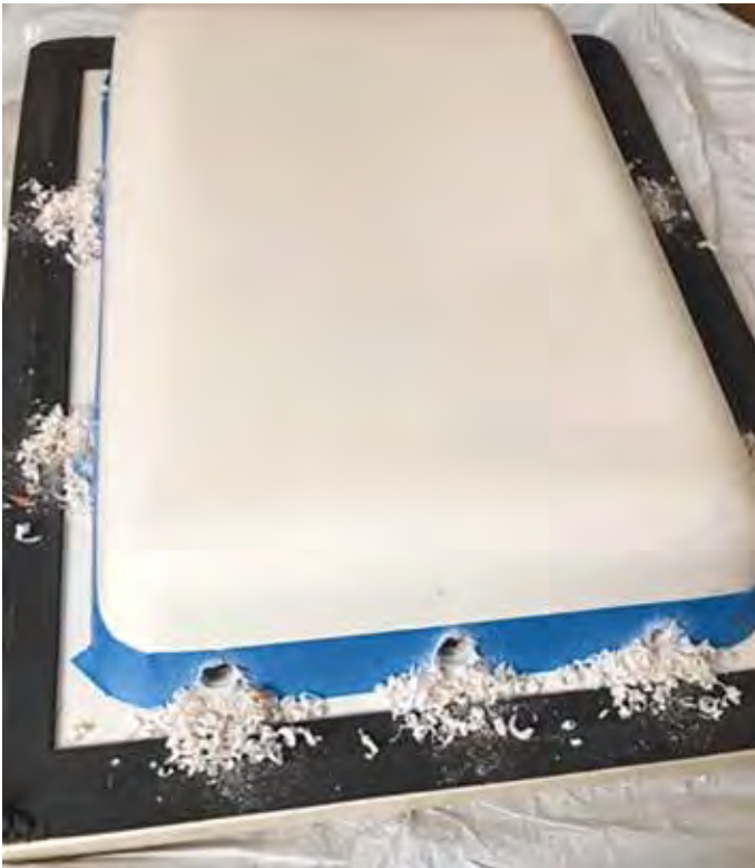
Locations of holes used to expose the void.
