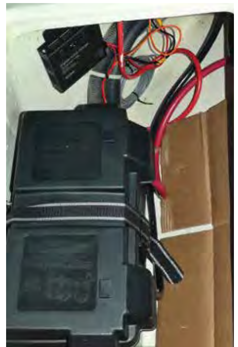
The SG200 was placed above the switch panel and utilized an existing cut out in the top back of the panel.
