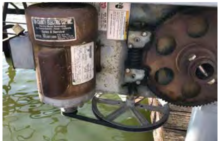
Original lift motor
