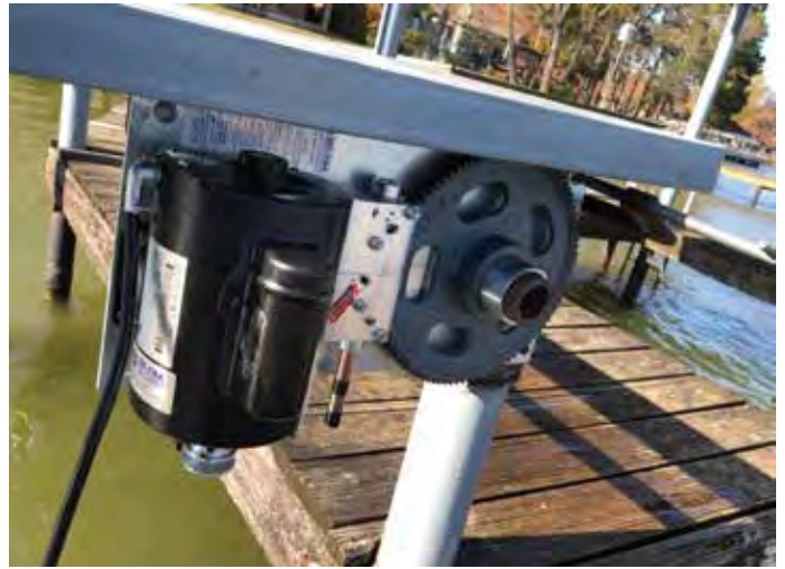
New lift motor
