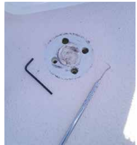
Mounting hole repair in progress. The area has been partially sanded to remove dirt and old sealant. One hole has been filled and partially redrilled. The others have been cleaned out using an allen wrench mounted in a drill.
