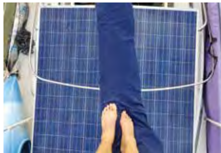
Additional 600W of solar power over the deck providing ample charging power.
