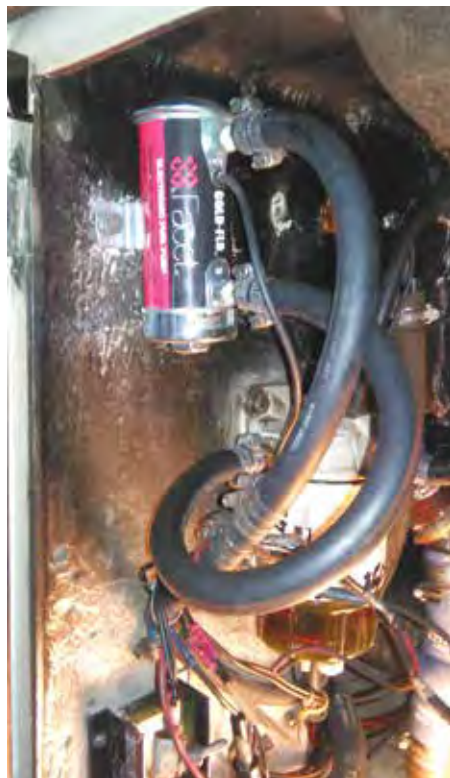
New Pump Location
