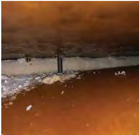
Port-side turning block between the deck and headliner. Exposed bolts are evident.
