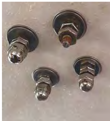
Interior acorn nuts removal reveals leaking
